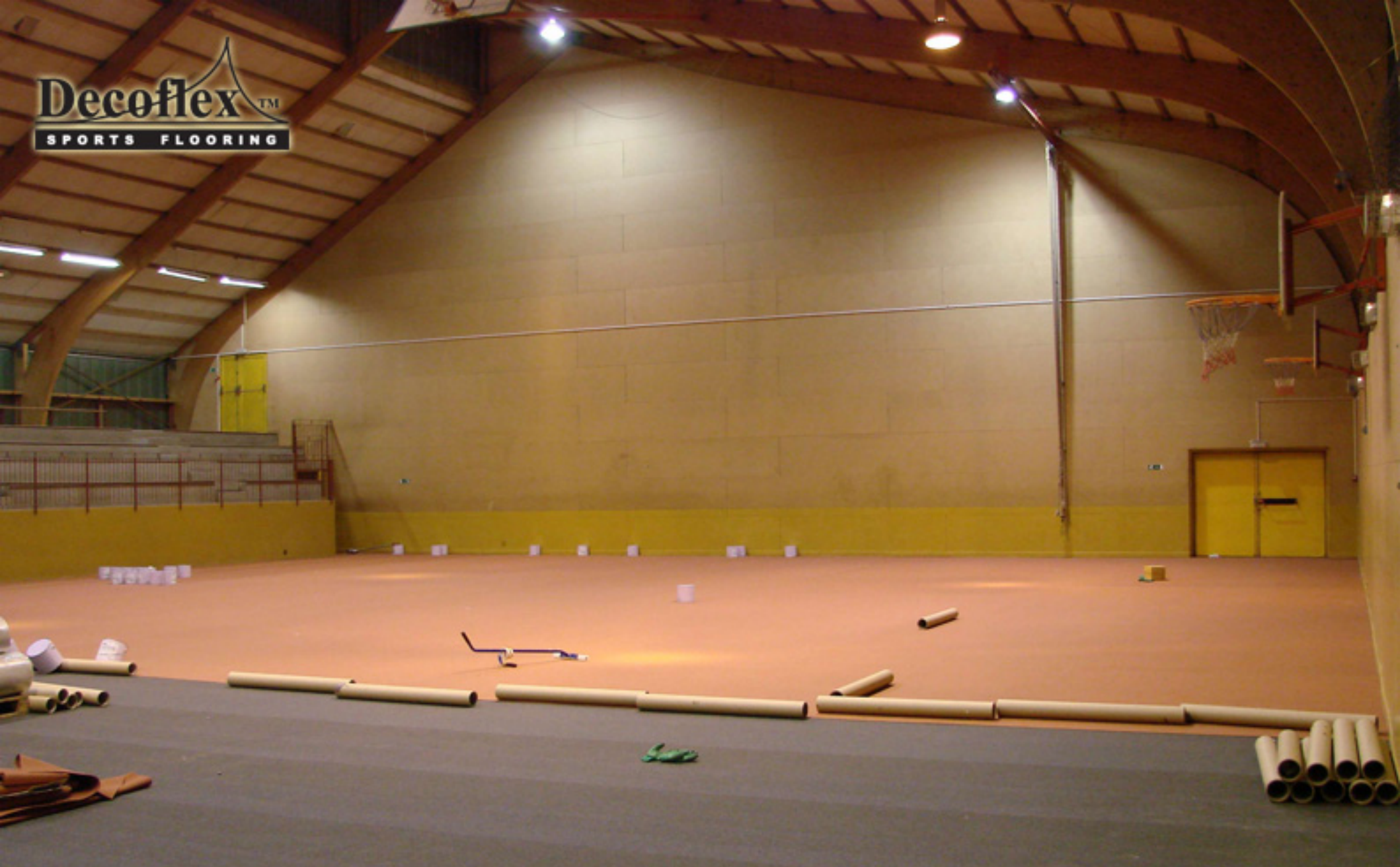
Decoflex 'D' Installation - EPDM Top Mat installed at 90° to the Base Mat
